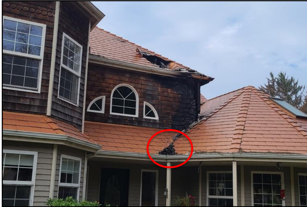
Figure 26. Attic fire started from roof/gutter debris and wildland fire (photo source: SCUF).
