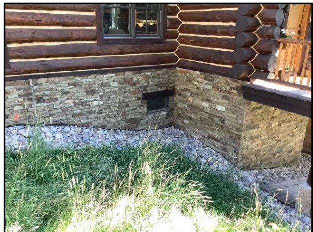
Figure 28. Non-combustible foundation material.
