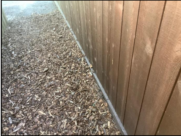
Figure 29. Combustible foundation material.
